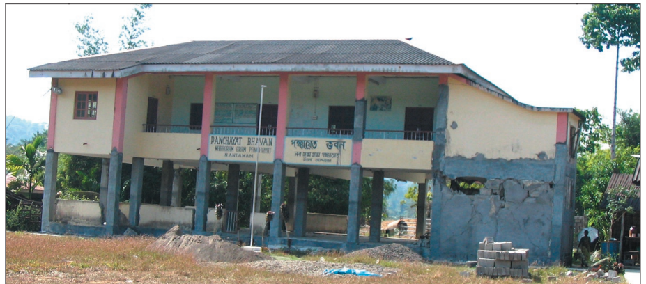
Figure 9a. The Panchayat Bhavan building showed severe cracking and damage to the soft first-story columns and infill walls (photo: Durgesh C. Rai).
