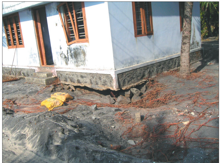
Figure 16. Scouring action at the base of houses due to returning wave of the tsunami in Kollam district in Kerala (photo: Alpa R. Sheth).
