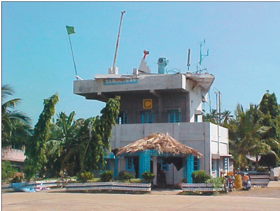
Figure 12a. Partial-collapse of the upper story of the air traffic control tower at airport on Car Nicobar Island (photo: C.V.R. Murty).
