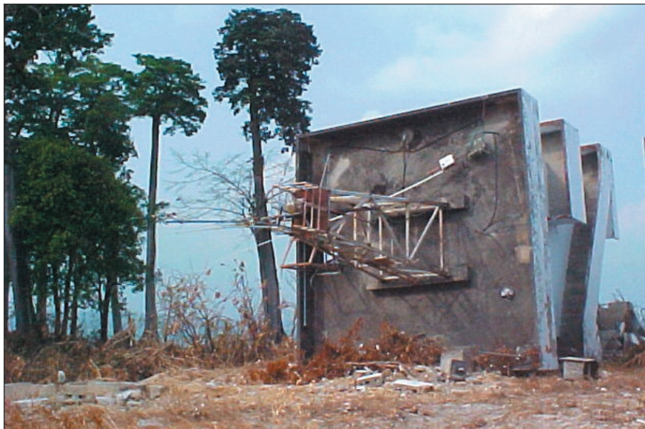
Figure 12b. Laterally toppled three-story seaport traffic control tower at Hut Bay in Little Andaman Island (photo: Suresh R. Dash).
