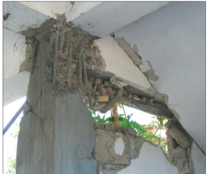
Figure 9b. Detail of column failure in the ground story (photo: Durgesh C. Rai).
