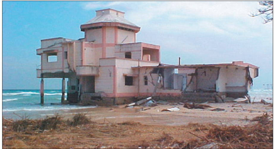
Figure 3. RC frame building (MES Inspection Bungalow) now stands in water on the eastern coast of Car Nicobar Island (photo: C.V.R. Murty).
