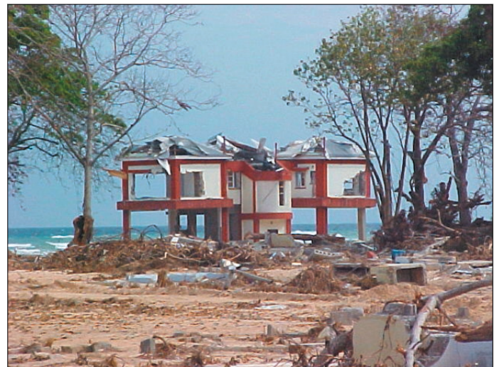
Figure 7. Shore-front building on Car Nicobar Island was inundated by the waves, but the frame resisted the wave effects (photo: C.V.R. Murty).
