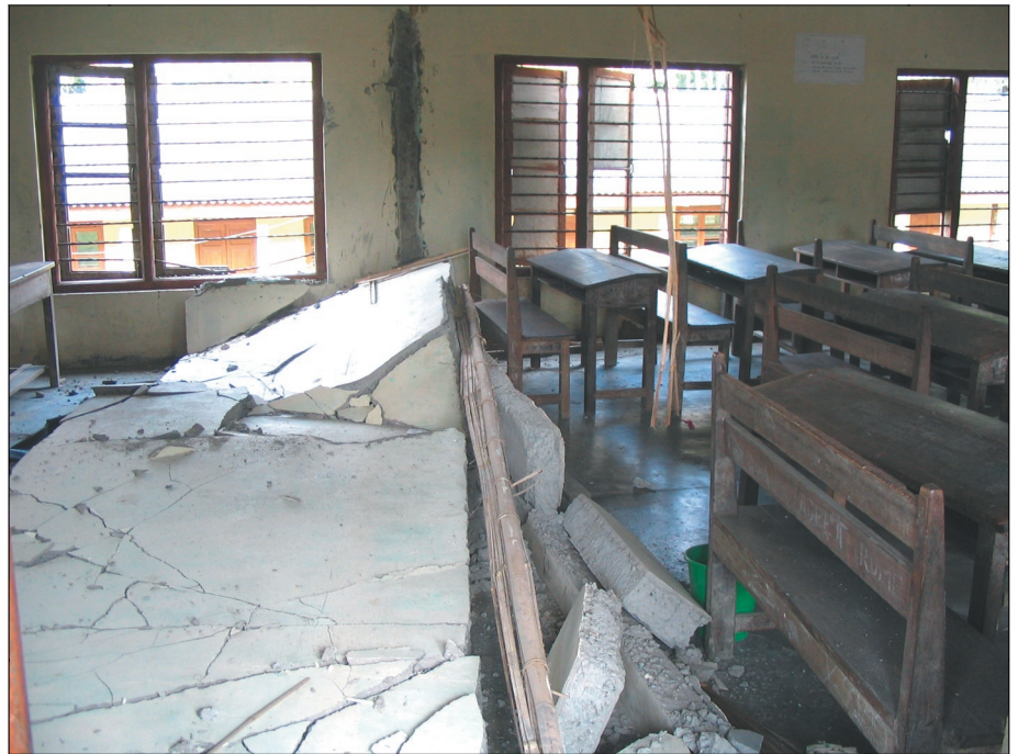
Figure 8. Slender masonry walls dislodged due to out-of-plane instability and poor or no connection to the surrounding structural elements (photo: Durgesh C. Rai).
