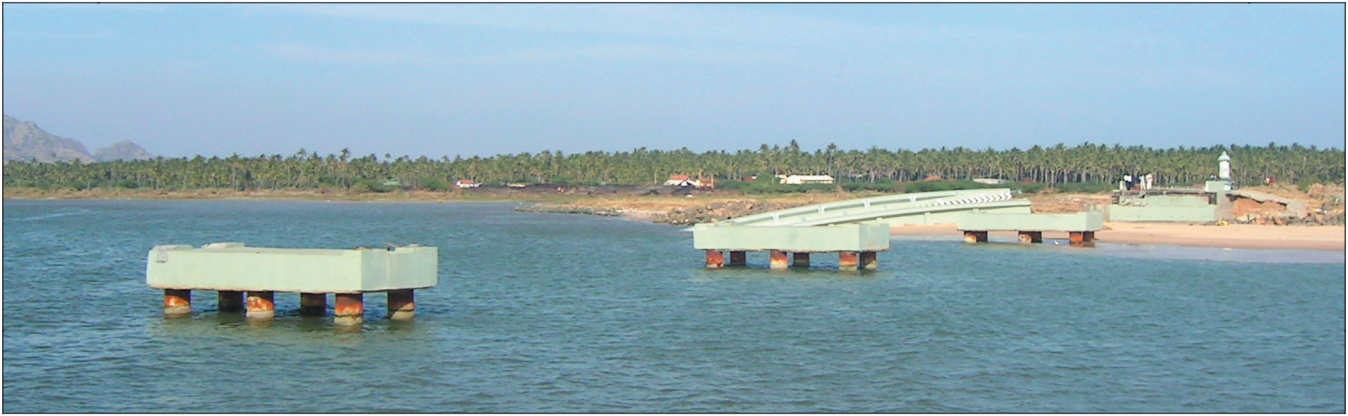
Figure 17. Complete loss of spans of the four span RC bridge at Melmannakudi in Tamil Nadu (photo: Alpa R. Sheth).
