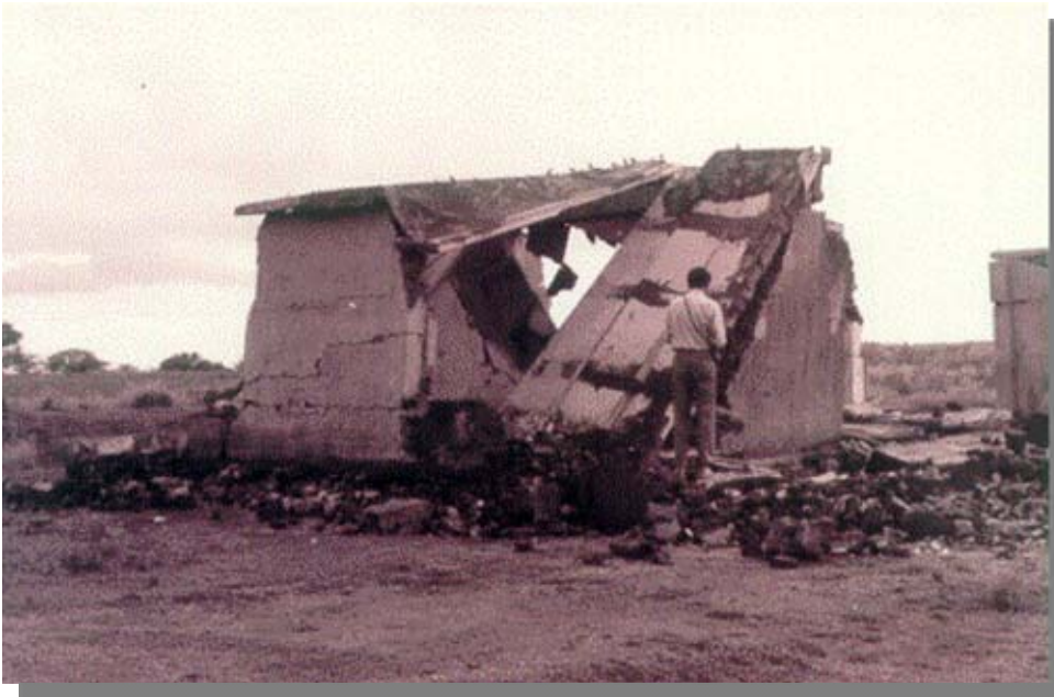
Figure 5: A brick masonry school building in Rajegaon collapsed. The roof of precast panels lacked adequate connections
