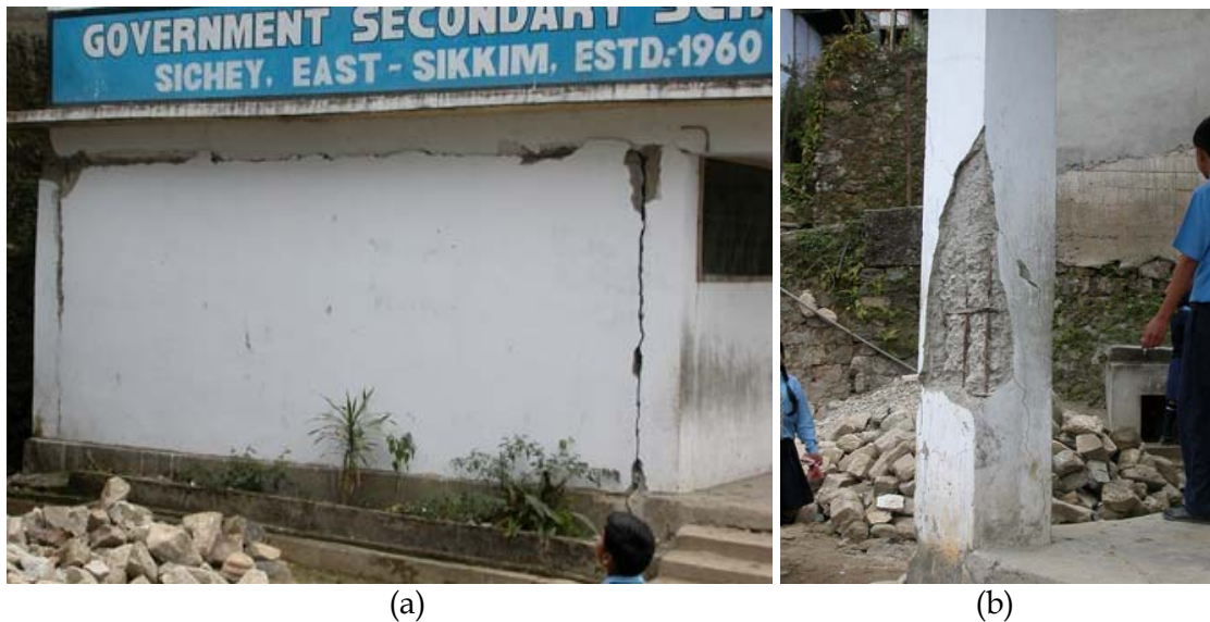
Figure 9: Government secondary school building at Sichey suffered moderate damages: (a) out of plane tilting of masonry infill wall, (b) inadequate shear reinforcement in columns, and spalling of cover concrete in columns at several locations due to corrosion.
