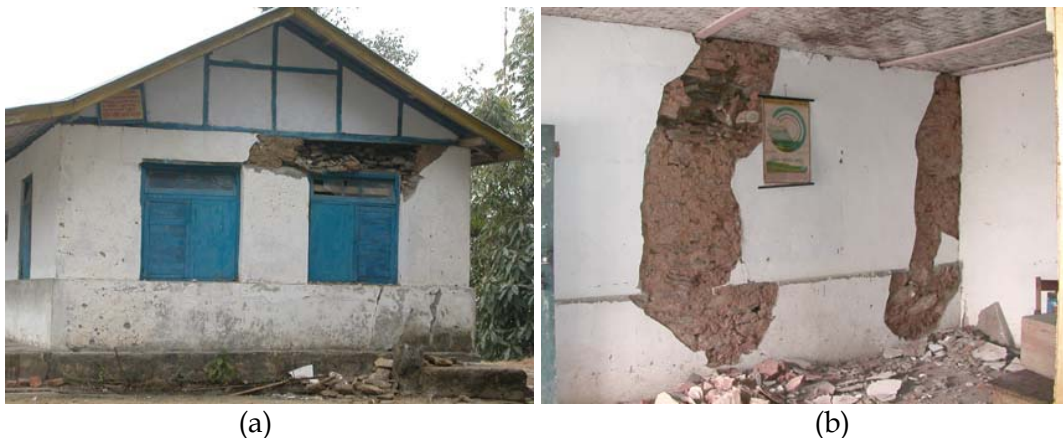
Figure 4: Severely damaged stone masonry low cost school buildings in Sikkim: Government primary school, Thamidara (near Gangtok).
