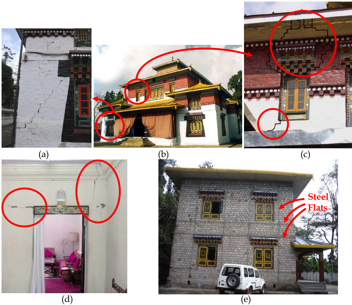
Figure 3: Performance of masonry structures at Gangtok: (a), (b), (c) wide shear and vertical cracks in masonry walls at corners and near openings in Enchey Monastery ; (d) numerous cracks near door/window openings were observed in Raj Bhavan ; and (e) good performance shown by retrofitted Archive building (arrows indicate locations of steel flats used to retrofit the building after 1988 Bihar-Nepal earthquake).
