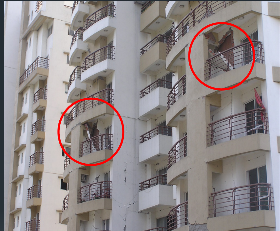
Combined in-plane and out-of-plane failure of infill panel
