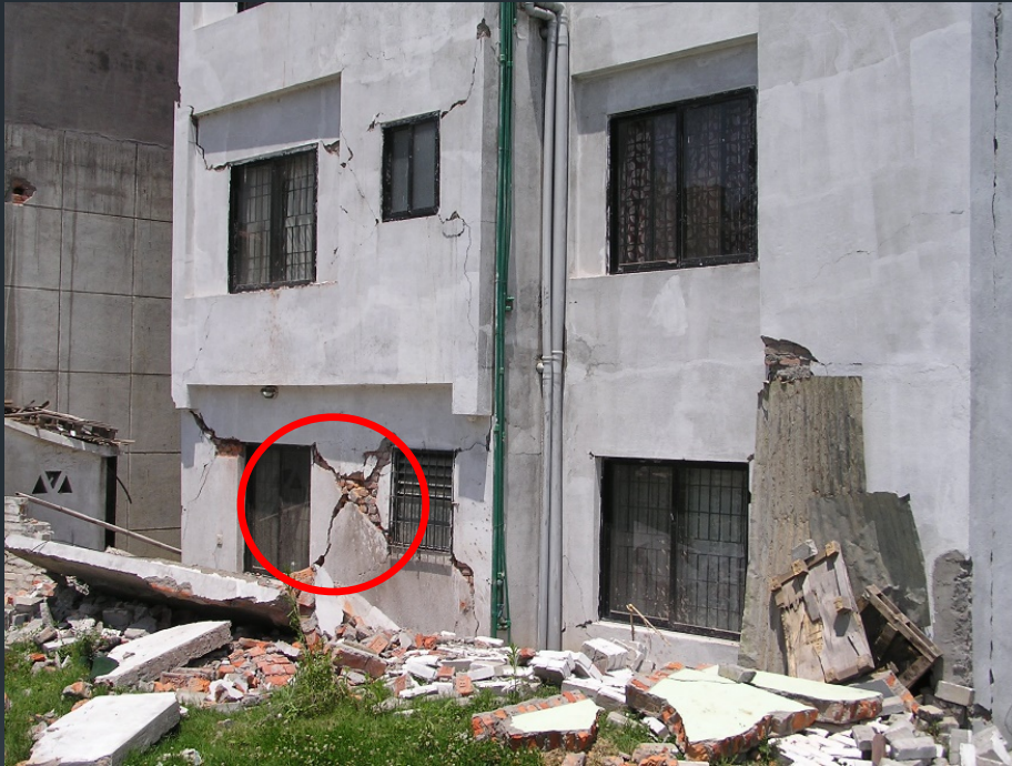
Diagonal cracks in the pier region between two openings
