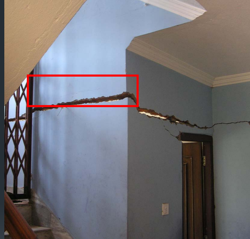
Horizontal crack in the infill wall due to differential settlement
