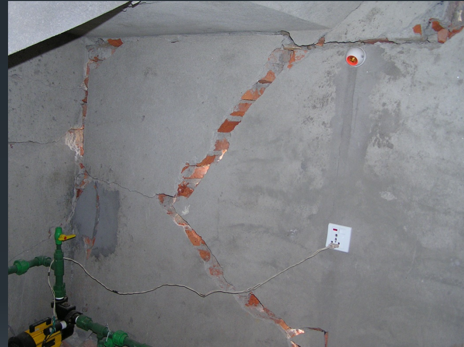
Inadequate strength due to use of half- brick thick infill
