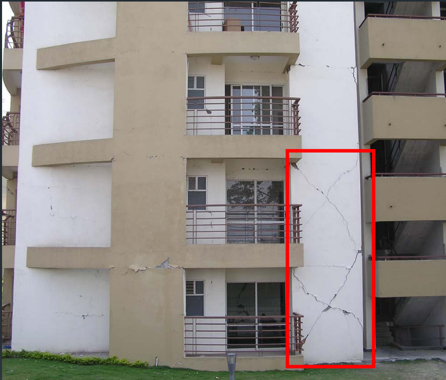
Diagonal cracks in the masonry panels
