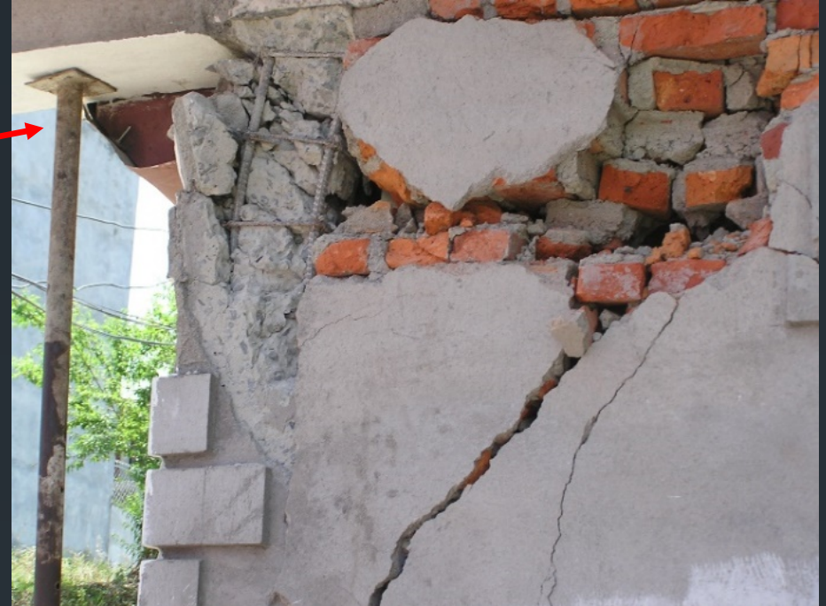
Masonry crushing and plastic hinge formation in column
