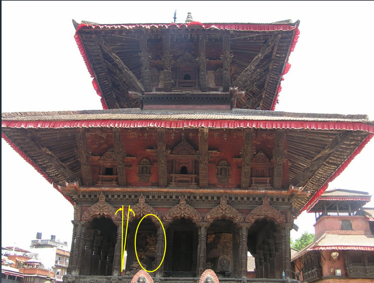
Sway of Timber frame and masonry collapse of Temple in Patan
