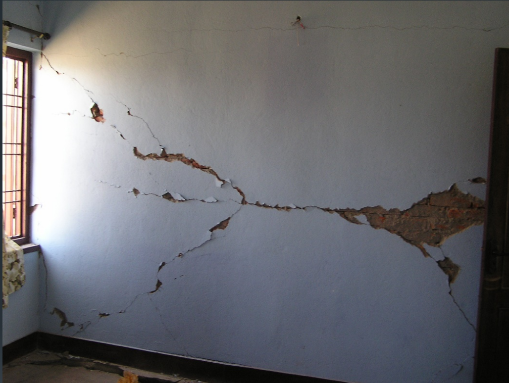
Diagonal and shear sliding crack at mid-height of wall
