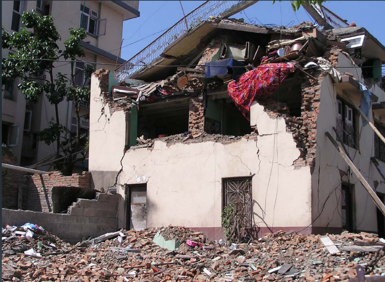
Pancake collapse of top storey of a 3 storey URM building, Kathmandu
