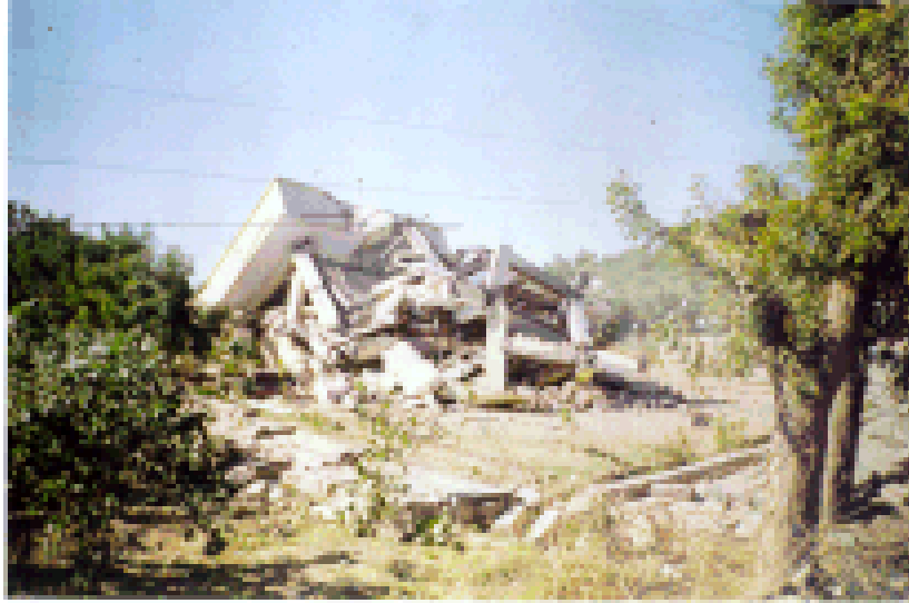
Figure 8.1 Failure of water tank in Manfera during the 2001 Bhuj earthquake
