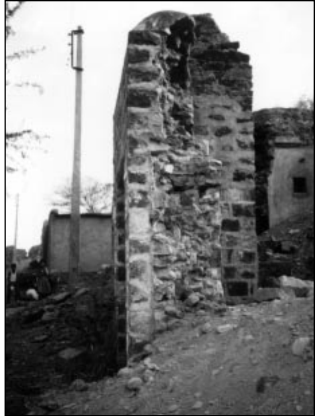
Figure 5 A typical stone wall with two exterior wythes and interior filled with rubble and mud (wall thickness over one meter).
