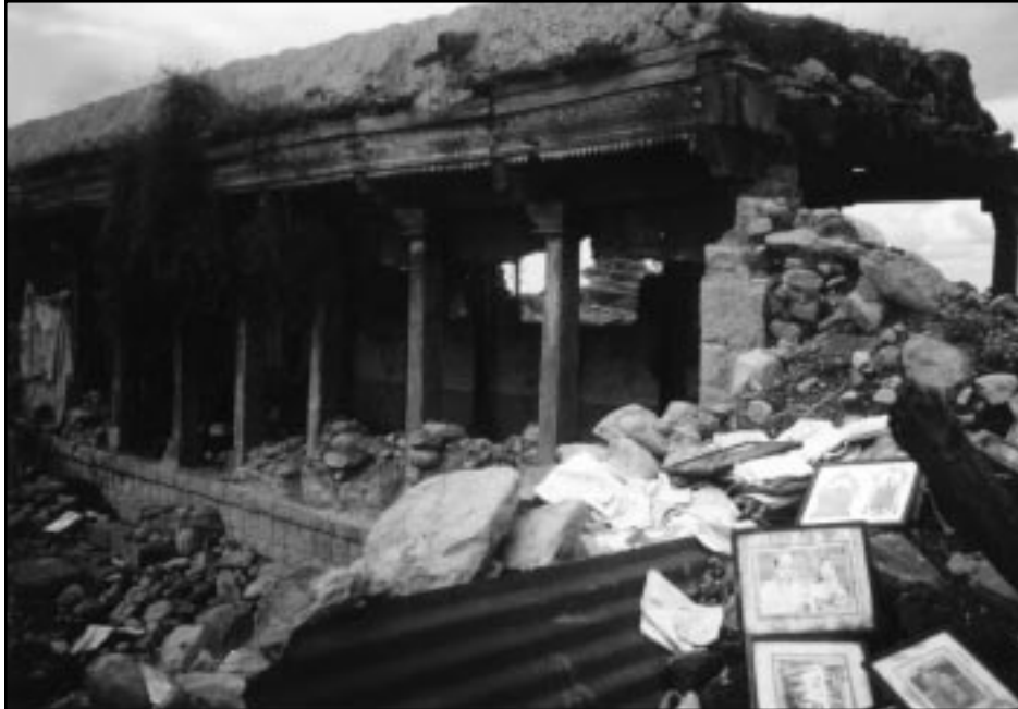
Figure 3 A typical timber frame with mud overlay in Killari village. The frame withstood the earthquake, but the walls collapsed.
