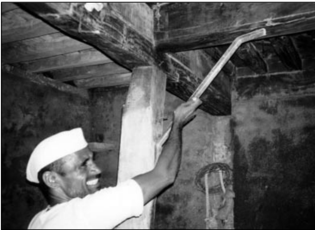
Figure 37 A beneficiary of the PSP showing a knee-brace used to retrofit a timber frame structure.
