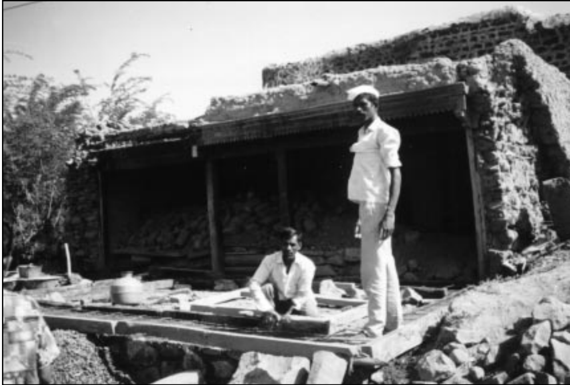
Figure 27 An example of a situation where retrofitting was not a feasible option due to excessive wall thickness and poor quality of construction. Masons are shown constructing a new plinth band.
