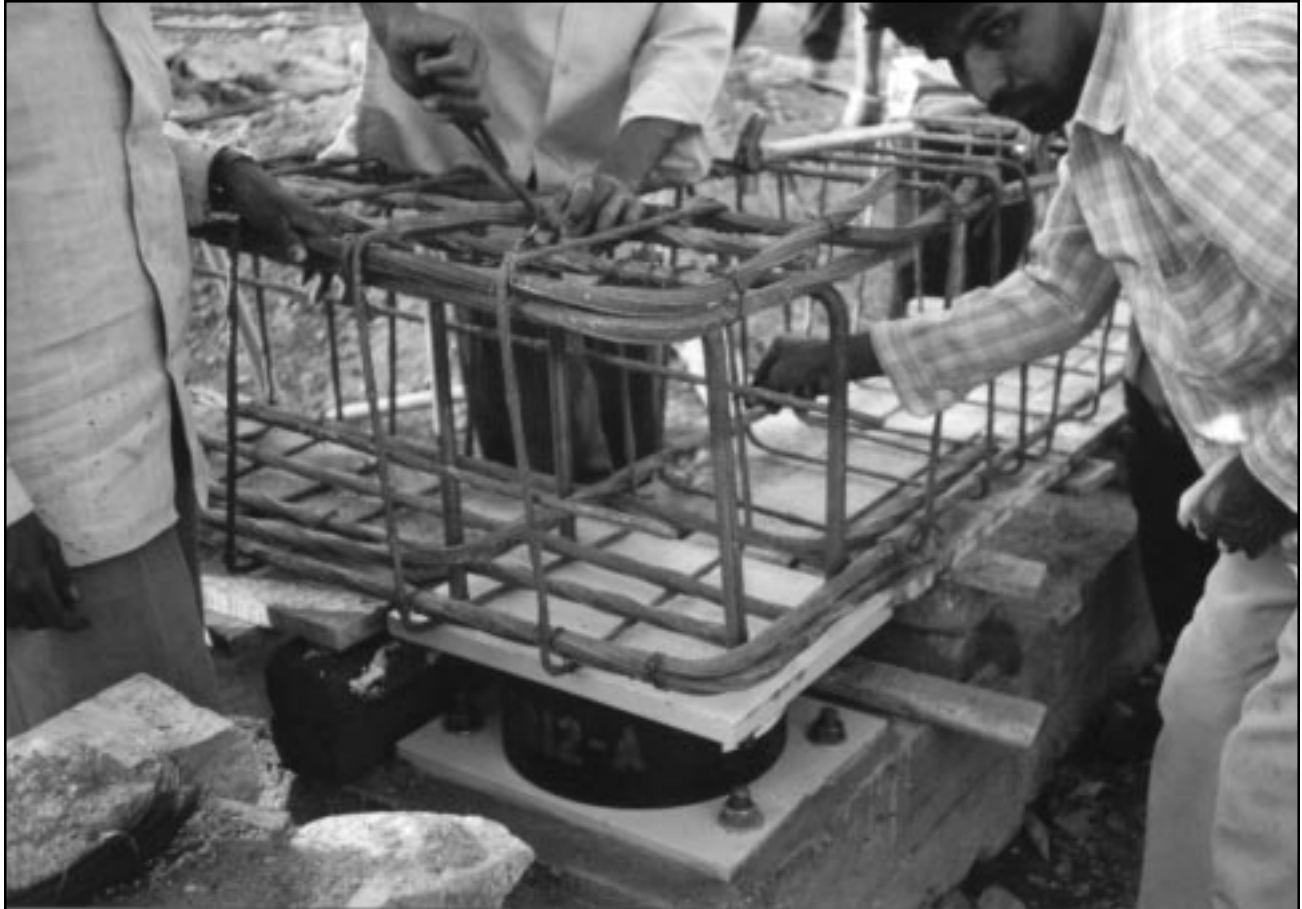
Figure 42 Construction of an upper concrete ring beam above the isolators for a school building in Killari village.
