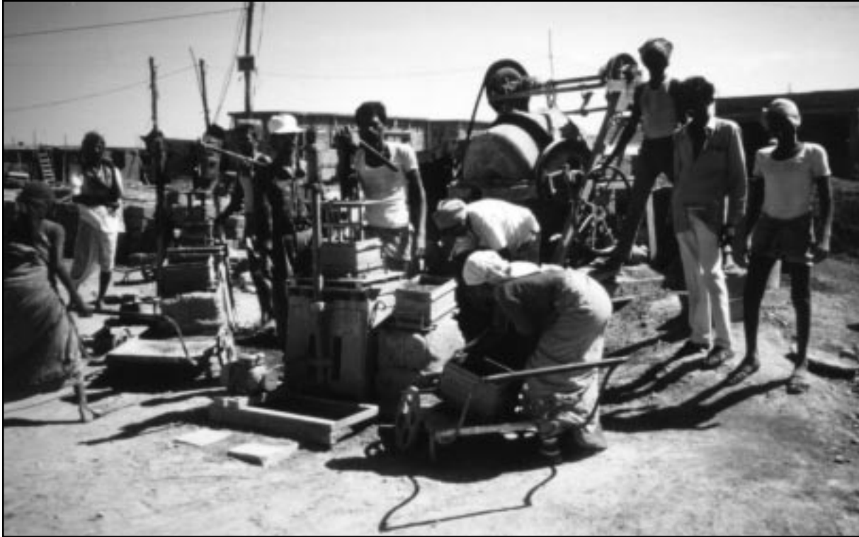
Figure 9 Manufacturing of concrete blocks by a contractor using a block-making machine in a relocation village.
