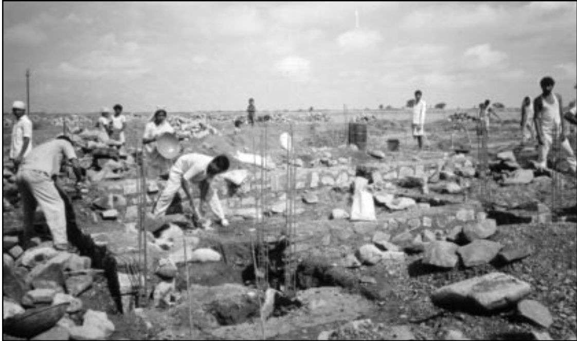
Figure 13 Construction of building foundations in Killari village. Stone masonry was used up to the plinth level.
