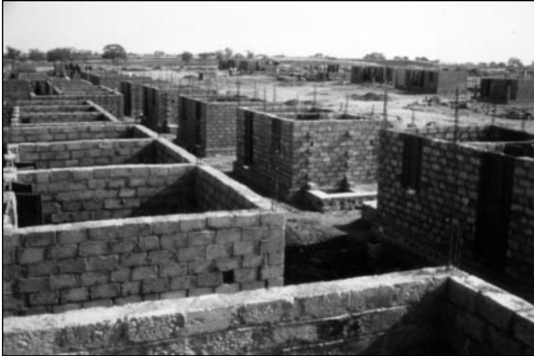
Figure 12 Vertical reinforcement bars were provided in concrete block wall construction (Killari village, Latur district).
