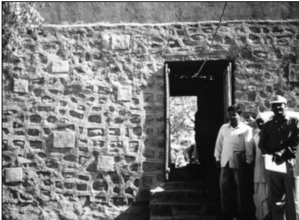
Figure 30 Junior Engineers inspecting a retrofitted stone house that has through-stones and a roof band.
