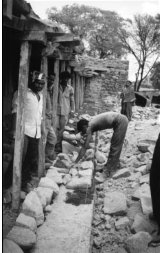
Figure 19 The GOM recommended reconstruction on the same plinth. The existing timber structure was preserved, and the walls were reconstructed in the improved manner.
