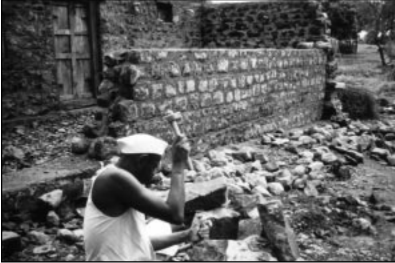
Figure 25 New stone walls were constructed using shaped stones cut by stonecutter artisans.
