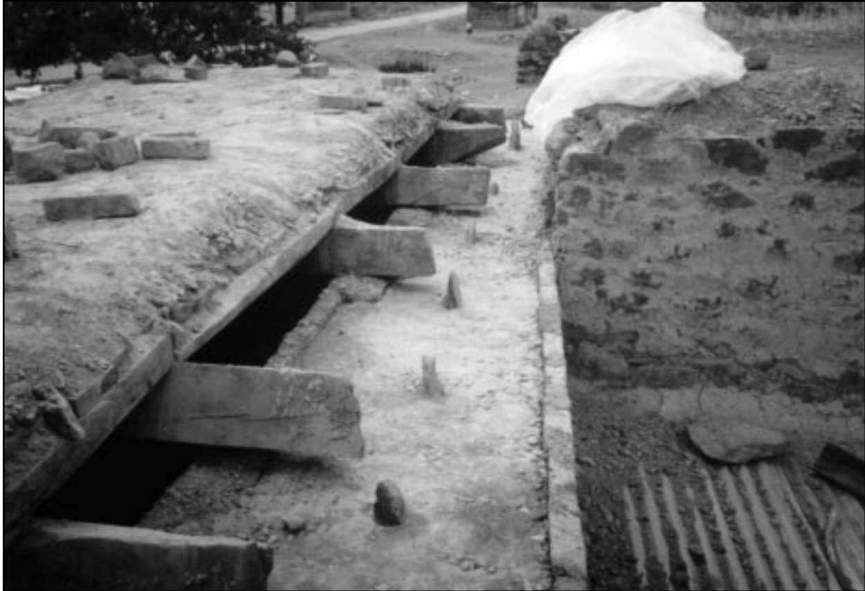
Figure 21 An example of concrete band installation at the eaves level of a stone masonry wall.
