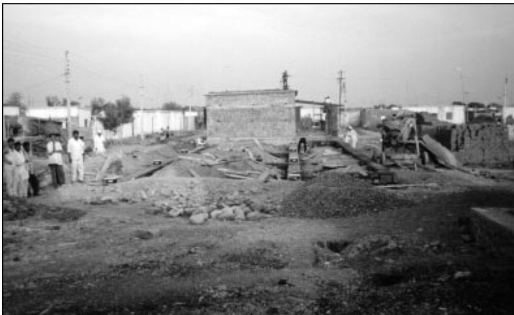
Figure 40 A half portion of the Killari school building was constructed as a base-isolated structure (under construction in foreground), and the twin brick masonry building in the background was constructed in a conventional manner.
