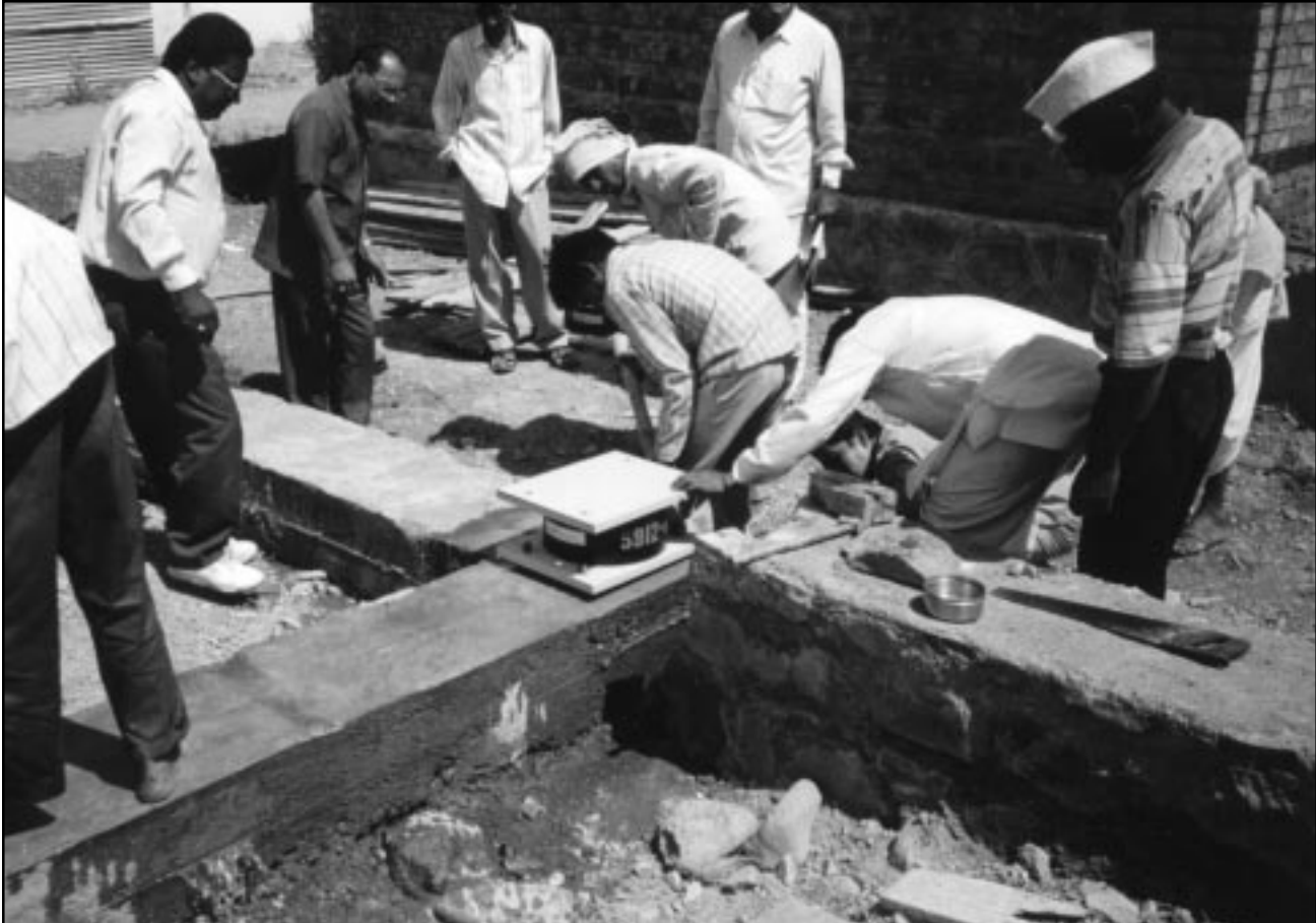
Figure 41 Installation of isolation bearings carried out manually using local artisans under the supervision of PMU engineers.
