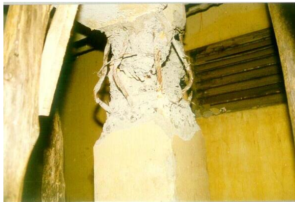
Figure 1 :: Damage to columns in Himgiri apartment.
