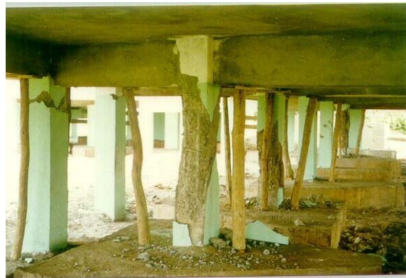
Figure 2 :: Damage to columns in the stilt storey of Youth Hostel building.
